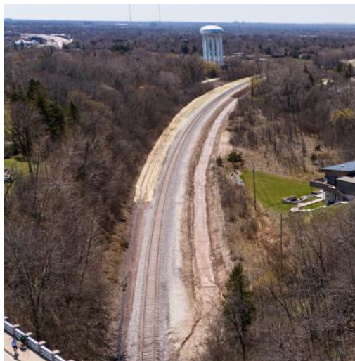
An aerial view showing Santa Monica Road on April 13, 2024. The track is in place on the new alignment. Photo by Mike Yuhás.
