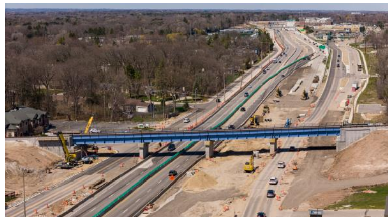
The new bridge, looking north, on April 13, 2024. The roadway between the west (left) abutment and the first pier is Jean Nicolet Road, two lanes. In the space between the first and second bridge piers are the temporary alignment of two southbound and two northbound lanes of I43; when road construction is complete, the three I43 southbound lanes will occupy this space. The northbound three lanes of I43 will be routed between the second and third piers. Port Washington Road is between the third pier and east abutment, and will be expanded to four lanes by the conclusion of the project. Photo by Mike Yuhás.
