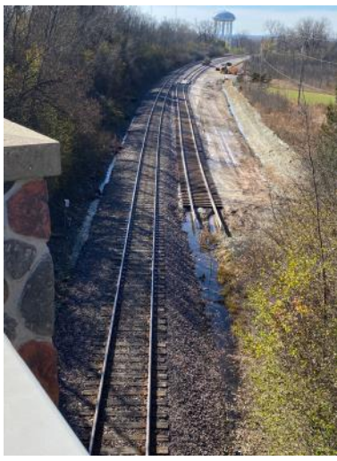
A similar view showing the new track alignment immediately to the north (right) of the existing track. November 19, 2023. Photo by Joe Kmoch.
